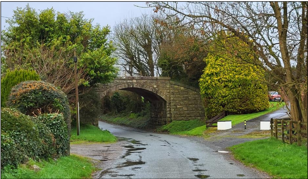
Figure 5.1.4.21d Stone bridge that carried the former L&NWR line over a local road
