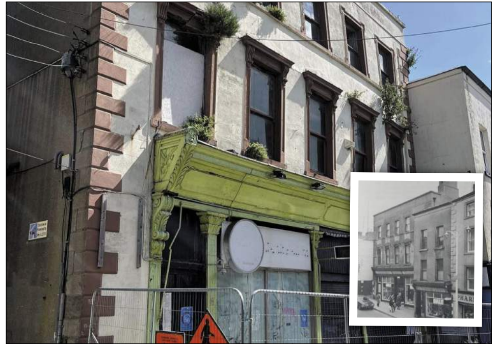
Masonry has been falling off the top floor of the former Brady's Department store building in Narrow West Street. Inset, Brady's in its former glory.
